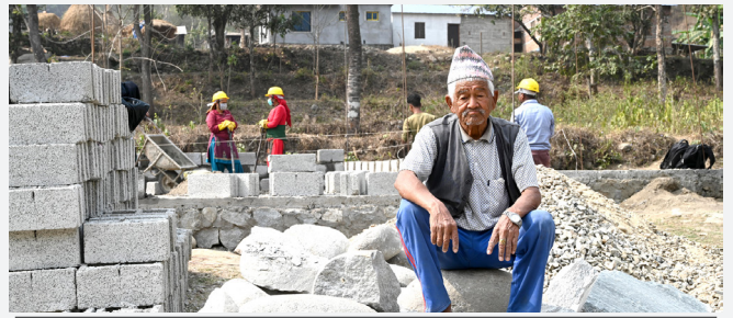
Dipa Bahadur Kunwar in the construction site of his house. Photo: Gajendra Shrestha
