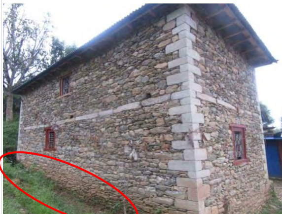
Absent of plinth beam
