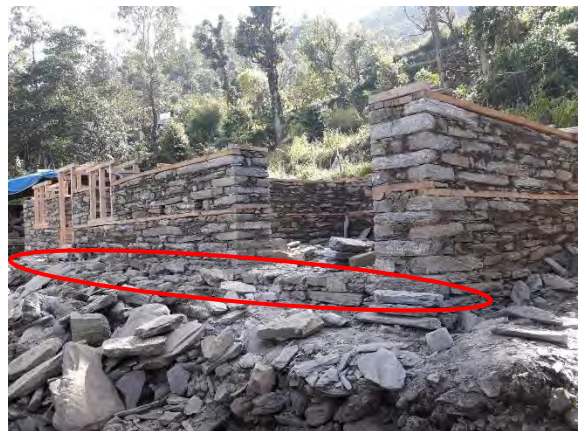
Absent of plinth beam
