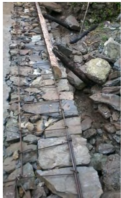
Inappropriate size of reinforcement
