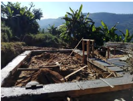
Absence of reinforcement at corner and T-junction.
