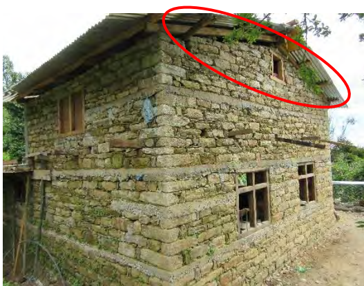
Unsupported gable wall
