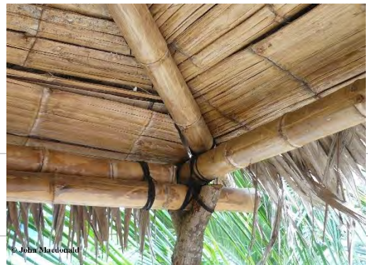
Vertical, Horizontal & Diagonal members connection using Lacing (Jute, Lylon, or equivalent) Techniques
