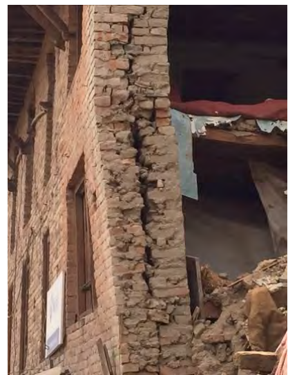
Delamination of wall
