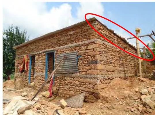
Unsupported gable wall
