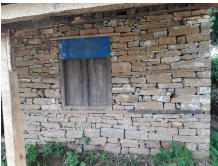
Absence of lintel band
