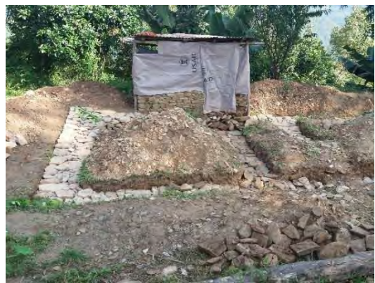
Shallow depth of foundation
